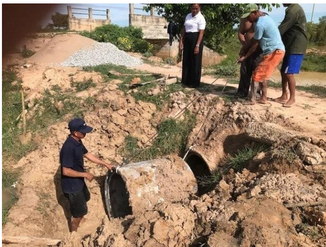
The culvert and canal will carry water for about one and a half miles to the dry paddies
